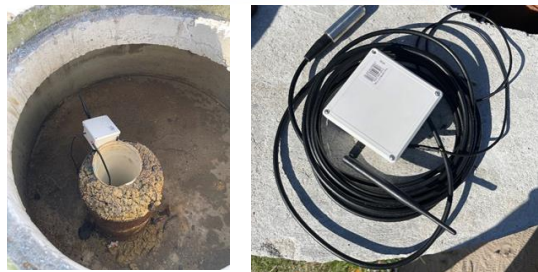
Hefei WNK8010 submersible water level sensor and node
