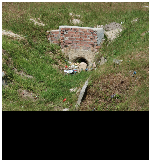
Figure C.6: Outlet structure with debris
